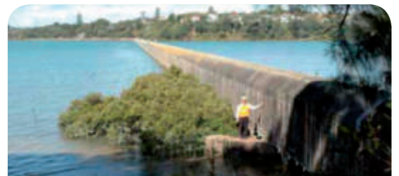
Like many of our large trunk sewers, the Hobson Bay pipeline is nearing the end of its life and is being replaced to provide more capacity
