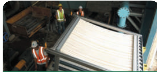
Membrane treatment technology
