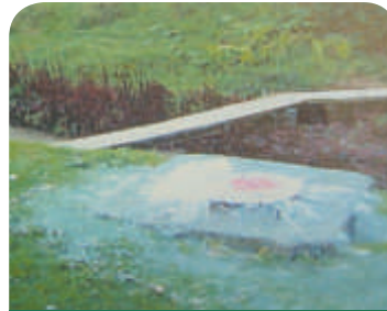
Unlimited wastewater overflows
