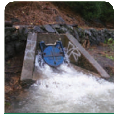
To avoid dry weather wastewater overflows that could occur almost daily in less than 30 years
