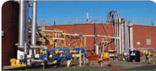
The Mangere Wastewater Treatment Plant is a state of the art facility which treats flows from Auckland City, Manukau City, Papakura District and Waitakere City
