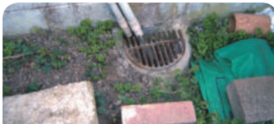
Gulley traps can allow large volumes of stormwater into wastewater networks
