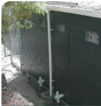
Many household and local wastewater pipes leak and overload the networks
